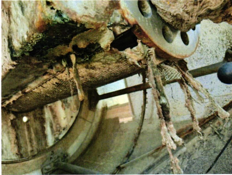
Figure 2. Damage to Fine Screening Unit
